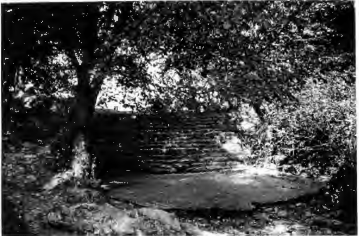
Figure 17. Dam 2. Note the concrete apron that has replaced the original apron. View is upstream.
