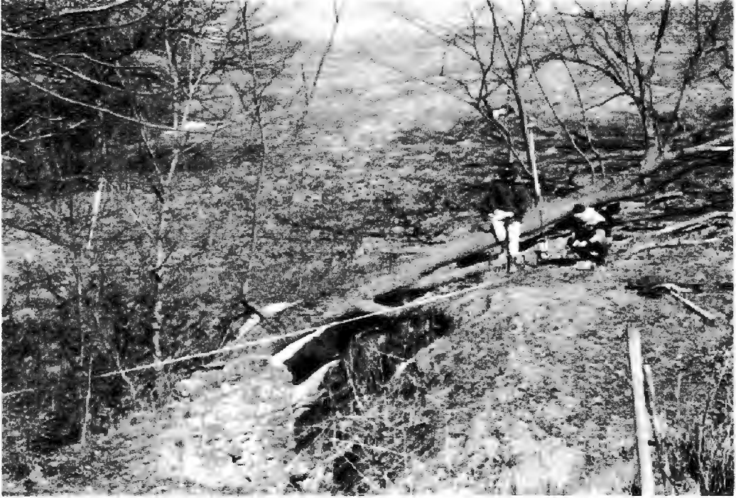
Figure 7. Destruction of the north side of Dam 1. The collapse of this tree forced the north side of the Dam into the middle of the gully.
