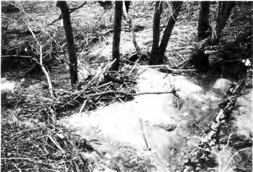
Figure 23. Debris on apron of Dam 3. Woody debris has formed a dam at the end of the apron that is trapping the large volumes of alluvial sand. View is from the southeast facing the northeast. Dam 3 is in the lower right portion of the figure.
