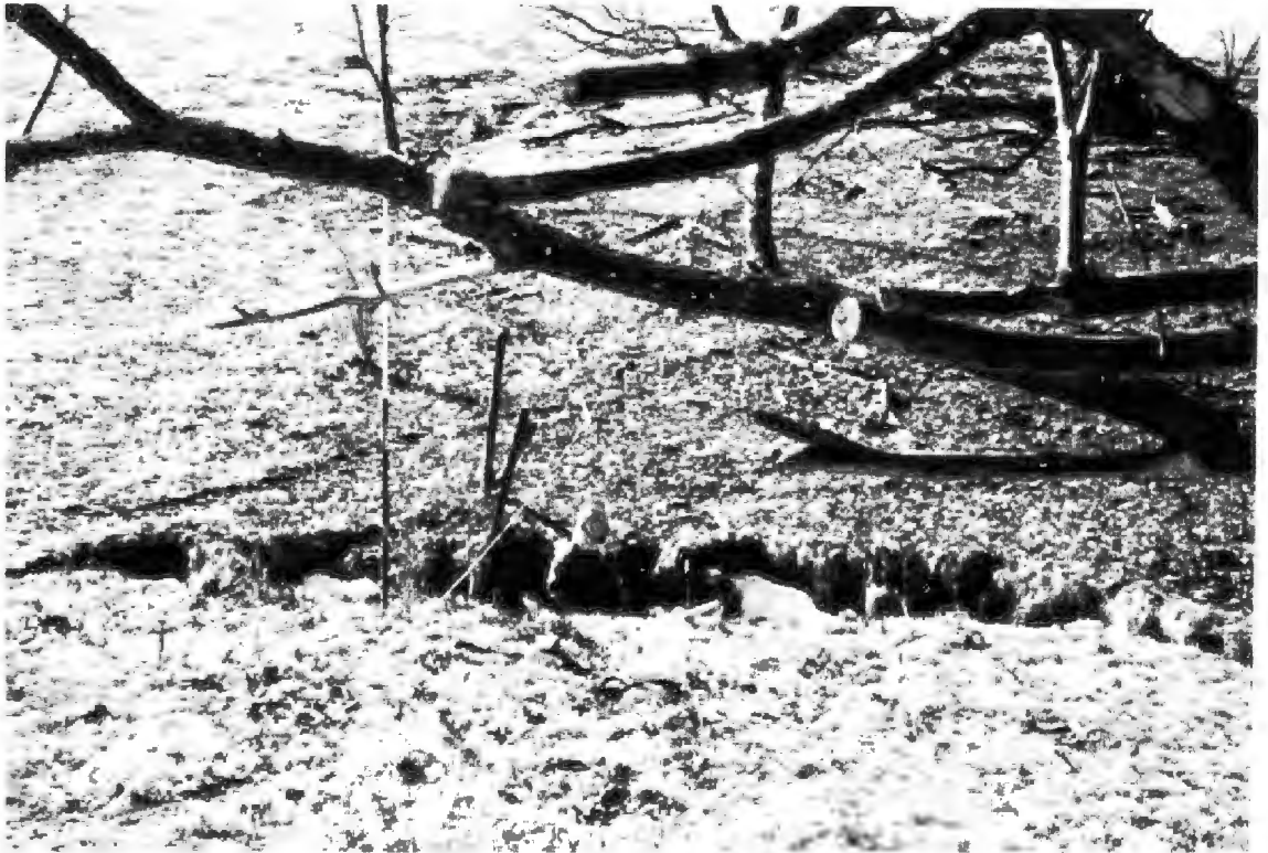
Figure 12. Extension of gully upslope of Dam 1. The headscarp of the gully is working its way upslope to the east (left). Dam 1 is just to the right of the photo.
