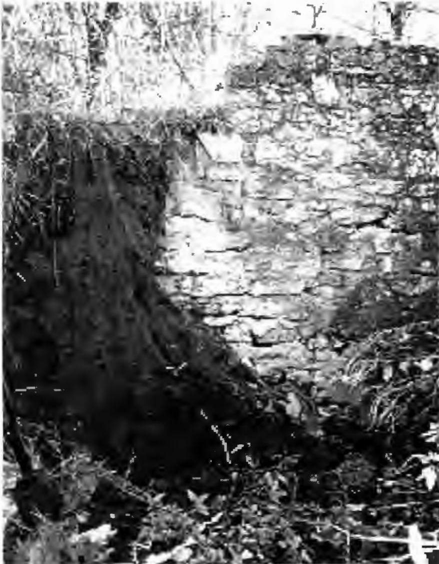
Figure 11. View behind Dam 1 facing downstream (west). Water is being deflected by the dam to the right of the figure (north) where it has eroded around the dam. Remnant historical fill can be seen to the left of the figure (south) underneath the abandoned spillway notch (top left of figure).
