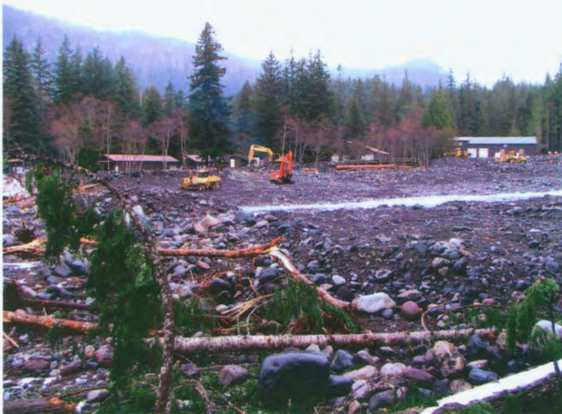
▲ FIGURE 6.9 Bulldozers and heavy equipment channelizing and altering the natural active channel of the Nisqually River at Longmire following November 2006 flooding. (Photo: Scott Beason, 11/21/2006)
