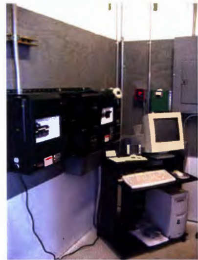
This image is of the computer based system that helps monitor and control the functions of the wind turbines and photovoltaic panels. Overall it is a very compact system.
