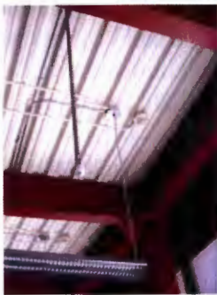
This image gives an even better feel of what the beam structure looks like as a painted finish as well as the texture of the ceiling.
