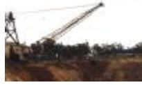
The machine that resembles a crane is used to remove the top soil.
