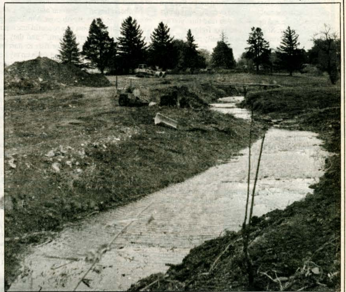
The demolition of the university golf course is finally in full swing. After years of speculation, the course was sold to the state last spring to allow the expansion of Highway 58 from a two-lane to a four-lane road from University Avenue to the relocated Highway 20.
