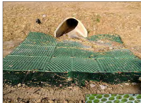
Flow transition mat, placed at culvert outlet over TRM on a prepared seedbed.
